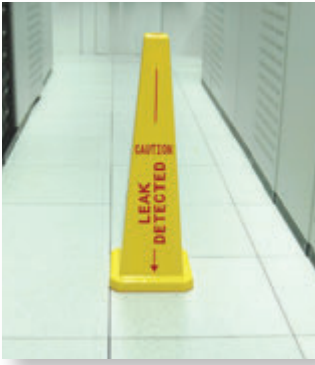
Water penetration poses a major threat to data centers, computer rooms, etc.
